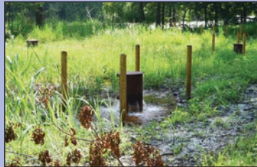
Buck Chute Relief Wells flowing
