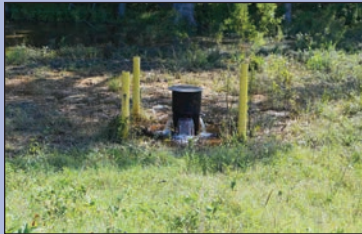
Above Greenville Relief Well Flowing
