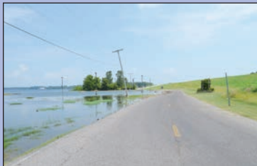
Greenville Boat Ramp Flooded
