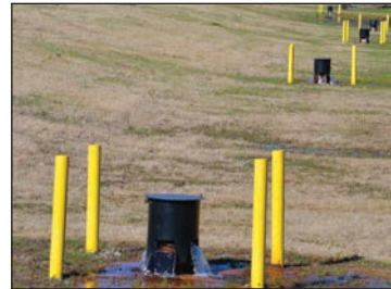
Above Greenville Relief Wells Flowing
