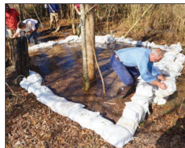
MS Levee Board Crew Building Sandbag Ring Around Sandboil at Ben Lomond
