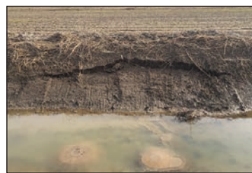
Sandboils in Valewood Ditch Near the Levee
