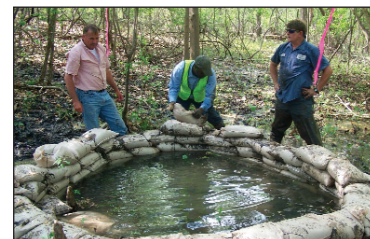
Sandbag Ring around Sand Boil at Buck Chute
